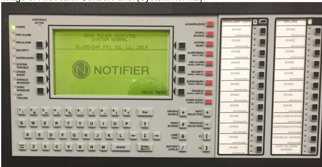
Image of Fire Alarm Control Panel (System Normal)
